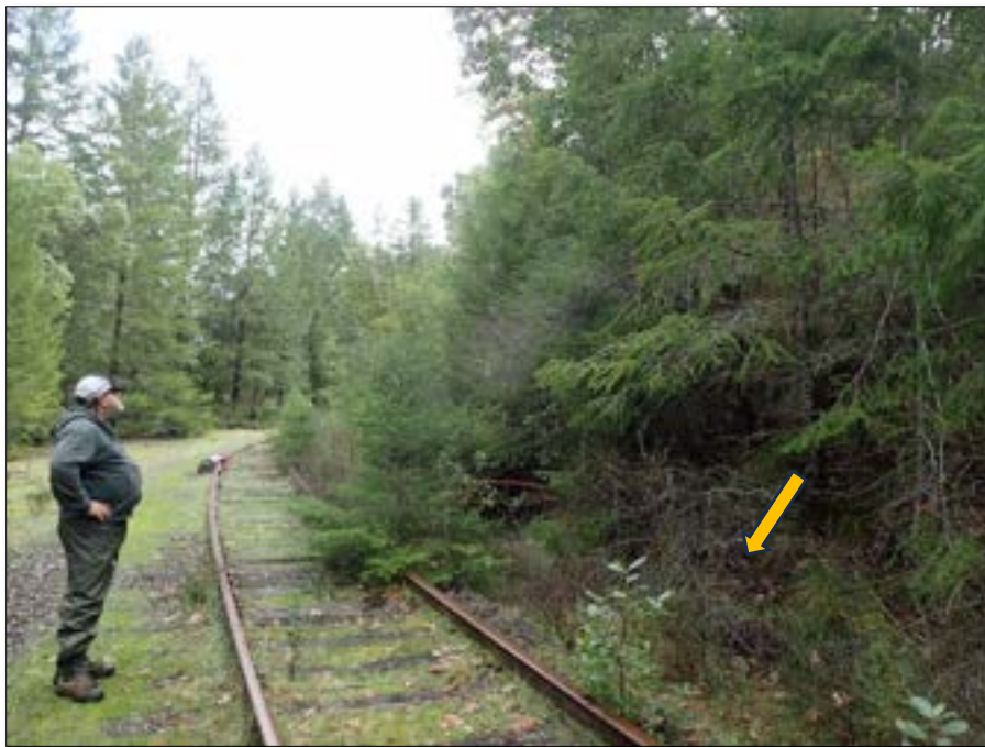
Photo 3. View of buried DRC at MM 132.5 located on the Great Redwood Trail approximately 4.5 miles south of Willits, California. Eroded sediment from a cutbank landslide deposit plugged the existing 18-inch diameter ditch relief culvert (DRC). Arrow shows vicinity of plugged culvert in inboard ditch with the thick brush. PWA recommends upgrading the existing DRC as the preferred alternative.
