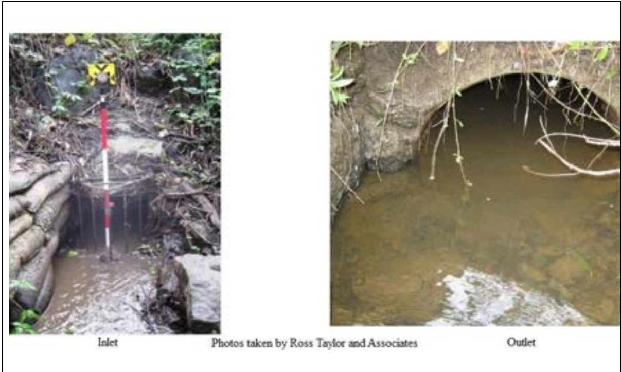
Photo 3 Photograph from CDFW's PAD for fish passage barrier ID number 765084, located on Jolly Giant Creek in Arcata.
