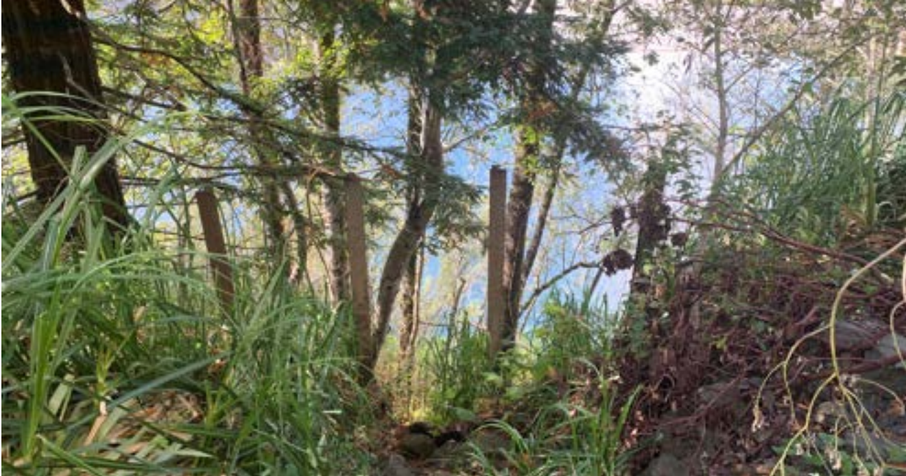
Washout of corridor with suspended track
