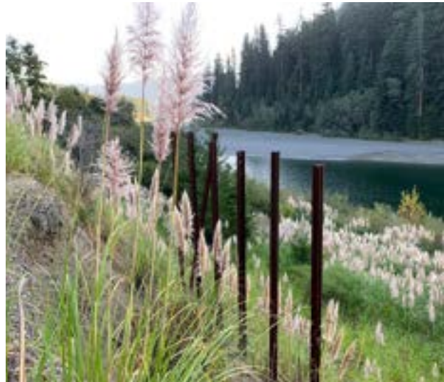
Failed wall along the Eel River
