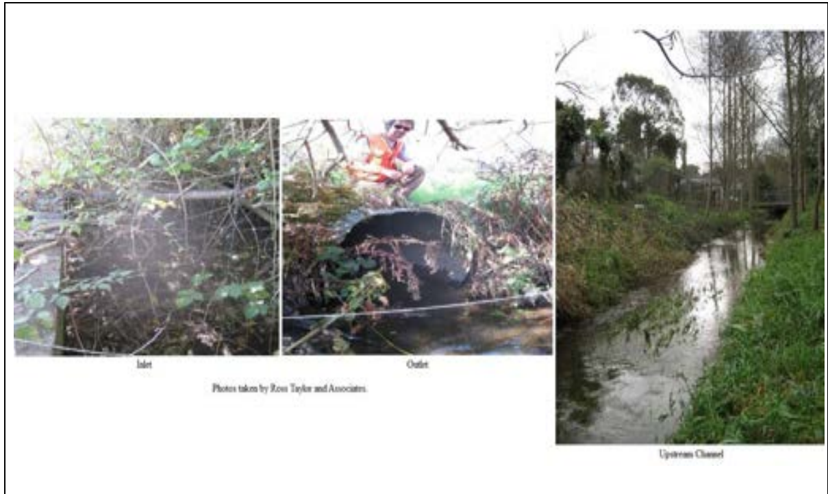
Photo 1 Photograph from CDFW's PAD for fish passage barrier ID number 765079, located on Jolly Giant Creek in Arcata.
