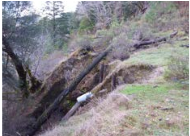
Culvert failures are frequent along the GRT and should be removed wherever possible to promote and restore natural drainage
