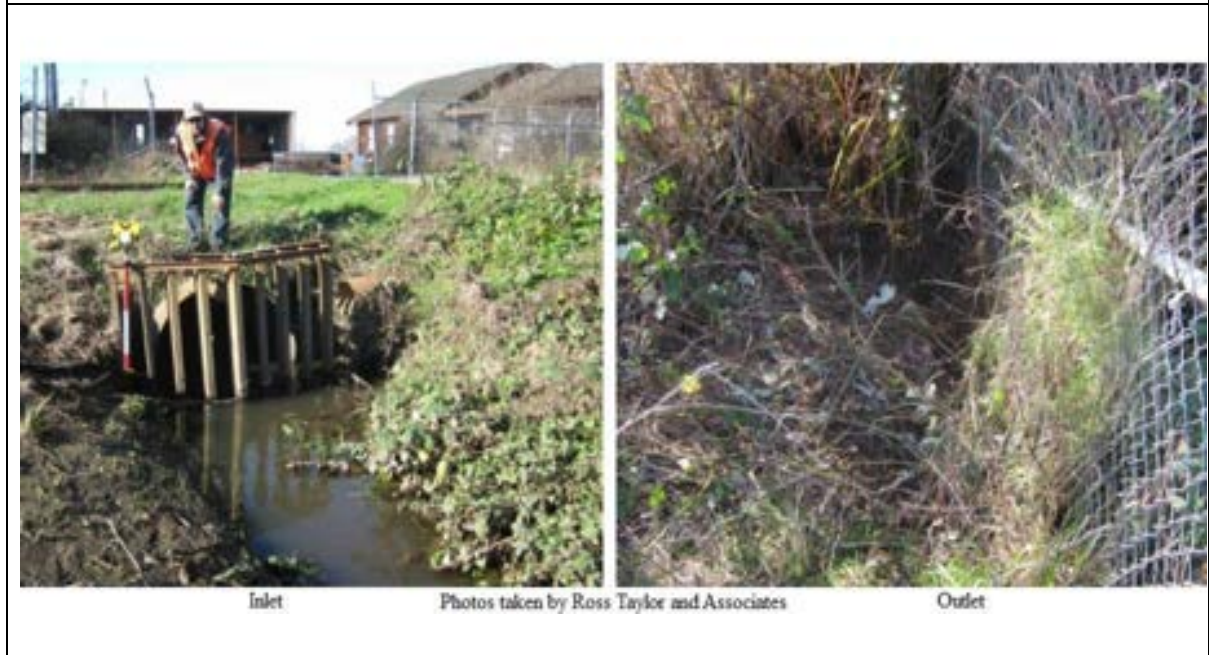
Photo 2 Photograph from CDFW's PAD for fish passage barrier ID number 765081, located on Jolly Giant Creek in Arcata.
