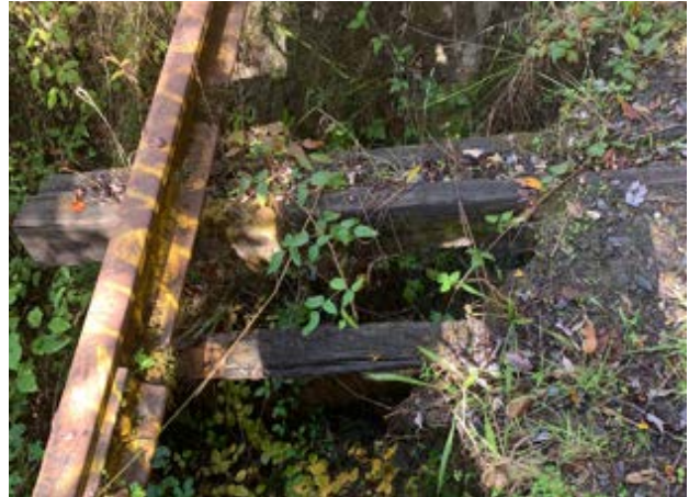
Existing failed culvert
