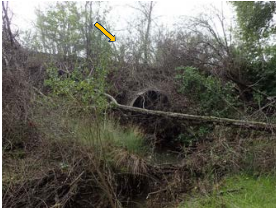
Photo 2. View of metal culvert outlet at MM 108.5 on the Great Redwood Trail. The channel has a relatively small scour hole at the culvert outlet, hydraulic forces during peak storms have eroded the stream channel bottom. Note geologist standing on the railroad alignment below arrow. This stream crossing culvert sized appropriately for 100-year peak stream flows and is functional.
