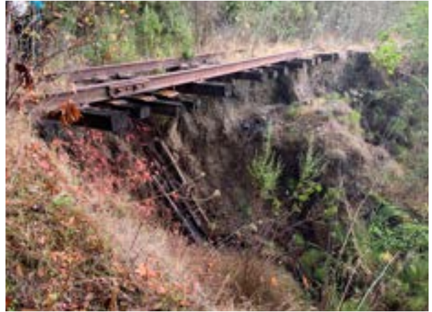
Existing failed culvert
