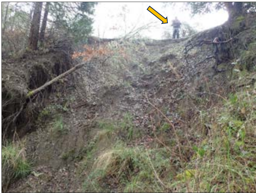
Photo 7. View of the fillslope failure and past erosion that occurred from the top of the railroad alignment to the base of the fillslope. Note the PWA geologist (yellow arrow) is standing on railroad alignment taking notes, conducting a rapid survey and sketching the existing conditions of the stream crossing site.
