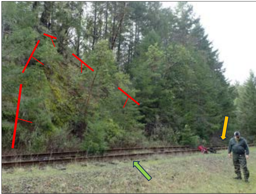
Photo 4. View of cutbank landslide (basic shape of main scarp is outlined in red) that plugged DRC (yellow arrow) and buckled tracks (green arrow) at MM 132.5 on the Great Redwood Trail. The cutbank landslide appears to have failed approximately 20 years ago based on the age of Douglas fir trees on the landslide deposit, which are 15 to 20 years old (basic shape of main scarp is outlined in red). The majority of the landslide is inactive, although a small rock fall occurred near the top in the recent past. The railroad tracks and wooden ties are slightly buckled and a little twisted.
