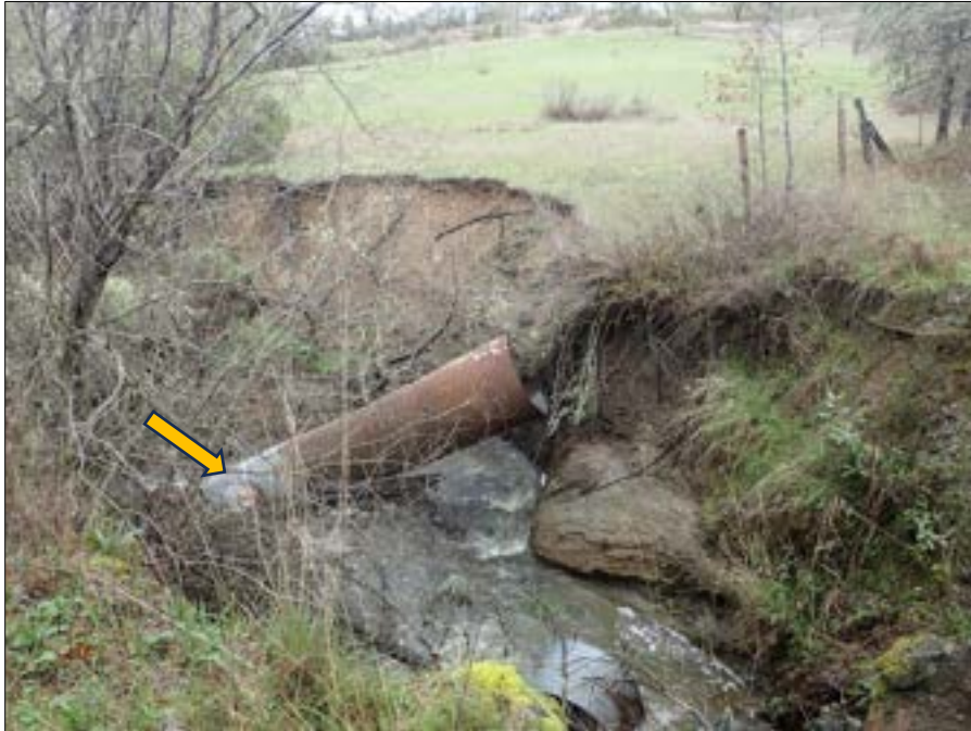
Photo 8. View of failed and separated culvert (yellow arrow) that lays dismantled and deposited in Walker Creek downstream of the railroad alignment. The separated and dislodged stream crossing culvert and significant volume of past erosion along the left stream bank makes this stream crossing site a high priority to upgrade.
