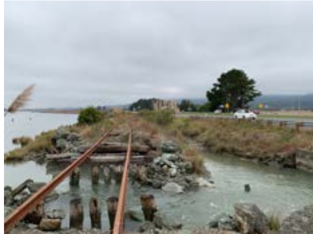
Failed trestle along Humboldt Bay
