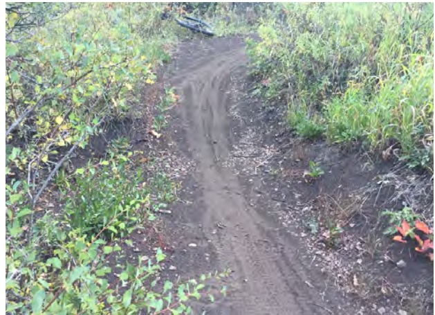
Dirt Crossings - drainage sheet flows across trail
