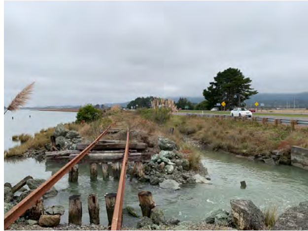
Failed trestle along Humboldt Bay
