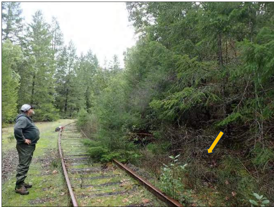
Photo 3. View of buried DRC at MM 132.5 located on the Great Redwood Trail approximately 4.5 miles south of Willits, California. Eroded sediment from a cutbank landslide deposit plugged the existing 18-inch diameter ditch relief culvert (DRC). Arrow shows vicinity of plugged culvert in inboard ditch with the thick brush. PWA recommends upgrading the existing DRC as the preferred alternative.
