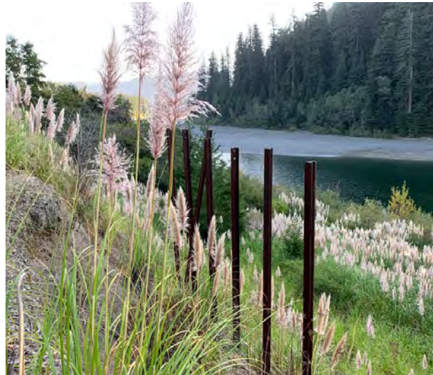
Failed wall along the Eel River
