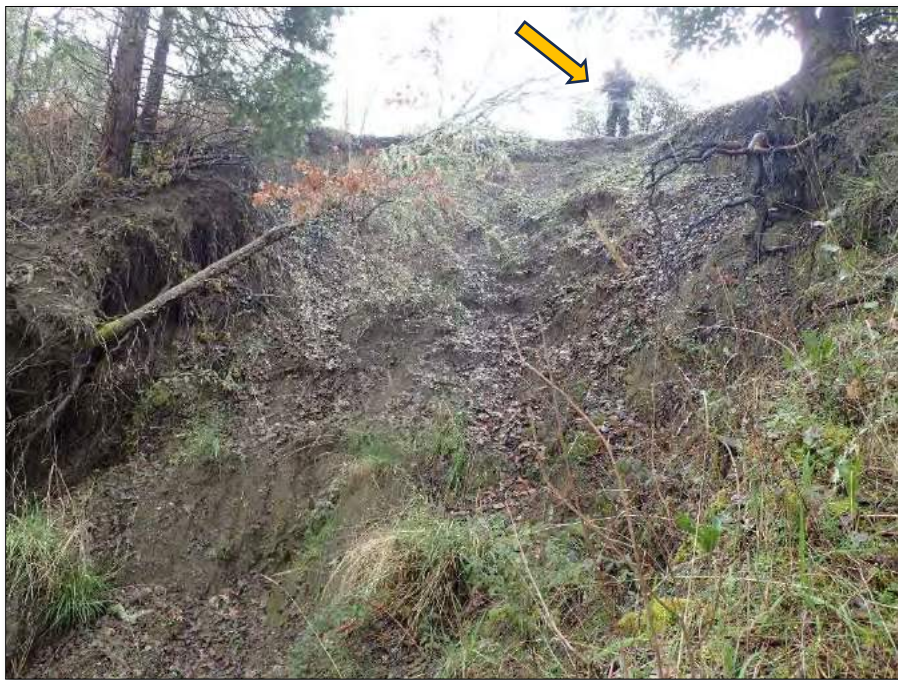
Photo 7. View of the fillslope failure and past erosion that occurred from the top of the railroad alignment to the base of the fillslope. Note the PWA geologist (yellow arrow) is standing on railroad alignment taking notes, conducting a rapid survey and sketching the existing conditions of the stream crossing site.
