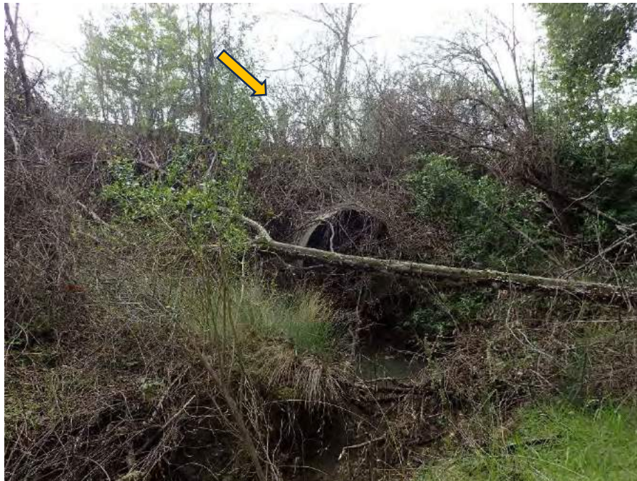
Photo 2. View of metal culvert outlet at MM 108.5 on the Great Redwood Trail. The channel has a relatively small scour hole at the culvert outlet, hydraulic forces during peak storms have eroded the stream channel bottom. Note geologist standing on the railroad alignment below arrow. This stream crossing culvert sized appropriately for 100-year peak stream flows and is functional.
