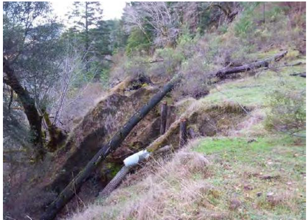
Culvert failures are frequent along the GRT and should be removed wherever possible to promote and restore natural drainage
