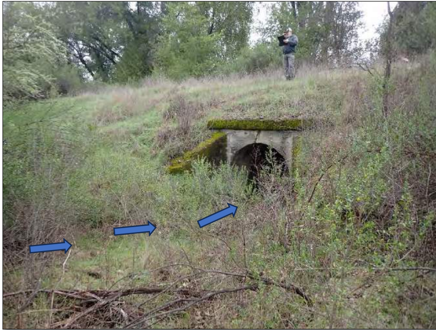
Photo 1. View of concrete culvert inlet at MM 108.5 a stream crossing culvert, on the Great Redwood Trail approximately 4.3 miles south of Ukiah, California. Arrows show flow direction. PWA estimated the 100-year peak storm flow rate at approximately 68 cubic feet per second (cfs) and determined that the existing culvert is properly sized to convey the 100-year peak stream flow including expected sediment and organic debris in transport.
