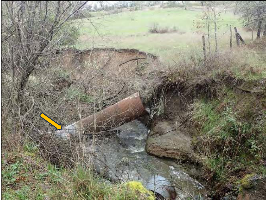
Photo 8. View of failed and separated culvert (yellow arrow) that lays dismantled and deposited in Walker Creek downstream of the railroad alignment. The separated and dislodged stream crossing culvert and significant volume of past erosion along the left stream bank makes this stream crossing site a high priority to upgrade.
