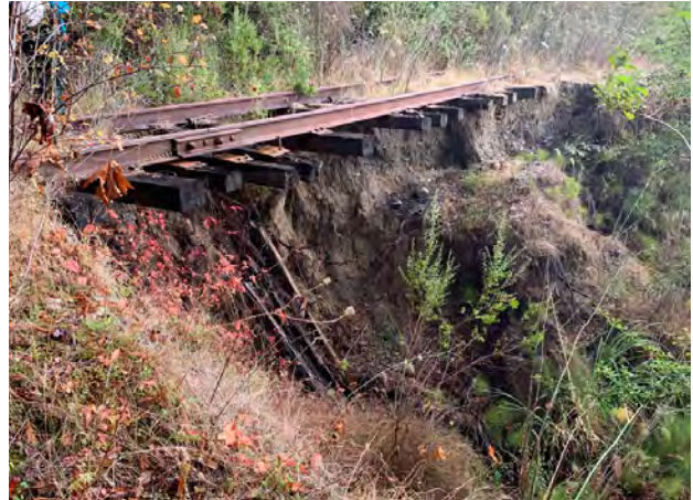
Existing failed culvert
