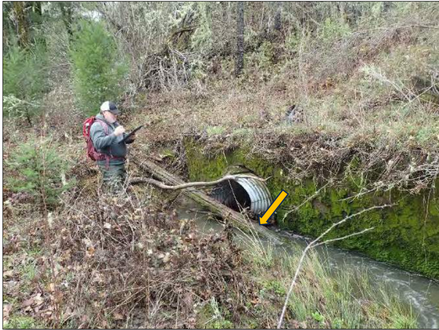
Photo 6. View of debris that blocked the stream crossing culvert inlet at MM 135.5 located on Walker Creek located on the Great Redwood Trail approximately 3.2 miles south of Willits, California. PWA's culvert sizing analysis determined that the culvert is not properly sized to convey the 100-year peak storm flow, including expected sediment and organic debris in transport. Arrow points to a log that floated into stream crossing and blocks culvert inlet.
