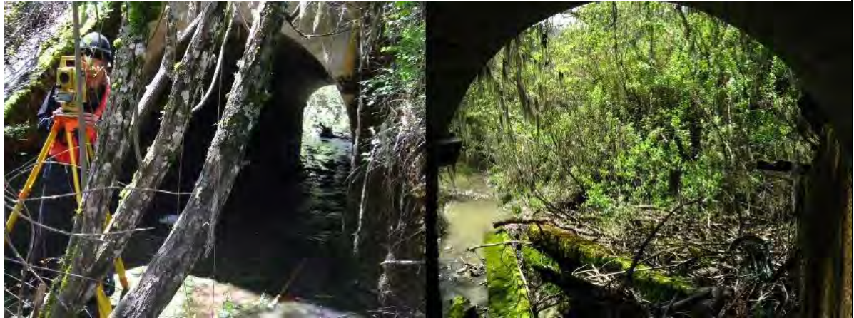
Photo 9 Photograph from CDFW's PAD for fish passage barrier ID number 758554, located on Haehl Creek south of Willits.
