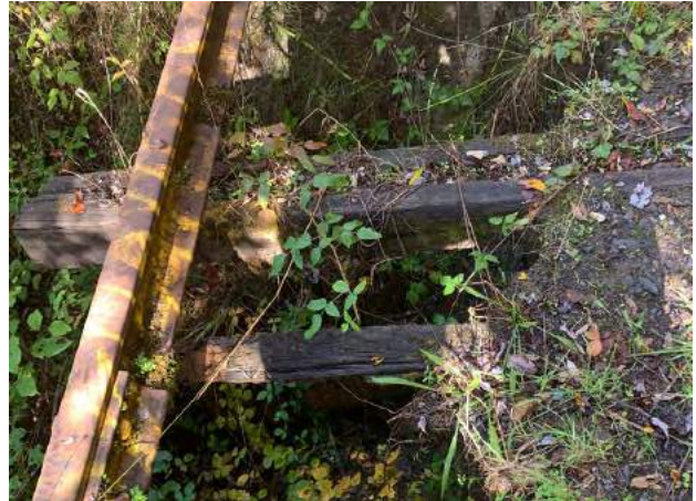
Existing failed culvert
